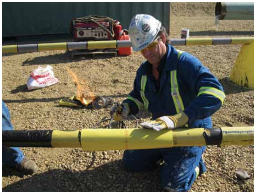
Among the technologies covered in the new NACE Pipeline Coatings Applicator Training Program is the application of heat shrink sleeves.
