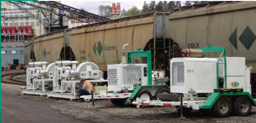
Four CCS owned UHP WJ pumps capable of deploying 6 guns and removing 240-1200 sq.ft. of coating per hour
