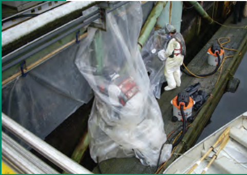
Chemical or shrouded vacuum tools can be cost effective when required for the deployment of spot abatement requirements.
