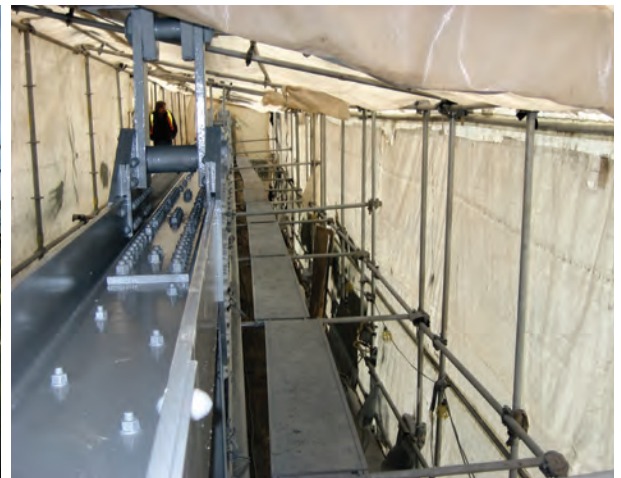
Liard Bridge - Sail Tarp containment to allow for the capture of blast media, paint overspray and the ability to control the work area environment.
